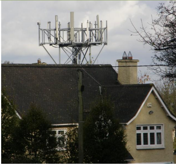
Transmitter Site Photo
